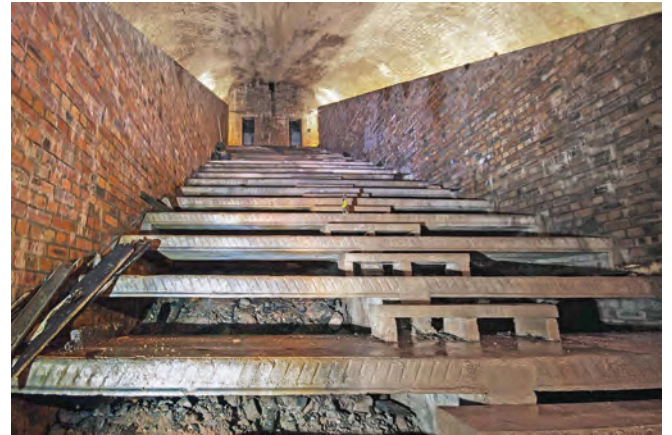
Lowermost shelter section 3 showing the precast concrete floor planks installed during the war when the centre level became an ARP shelter. Wartime blast walls form the sides with the access stairs on both sides behind them. The slenderest volunteers have been able to squeeze between the floor planks to search for relics dropped by the shelterers on the floor on which the original railway tracks were laid
